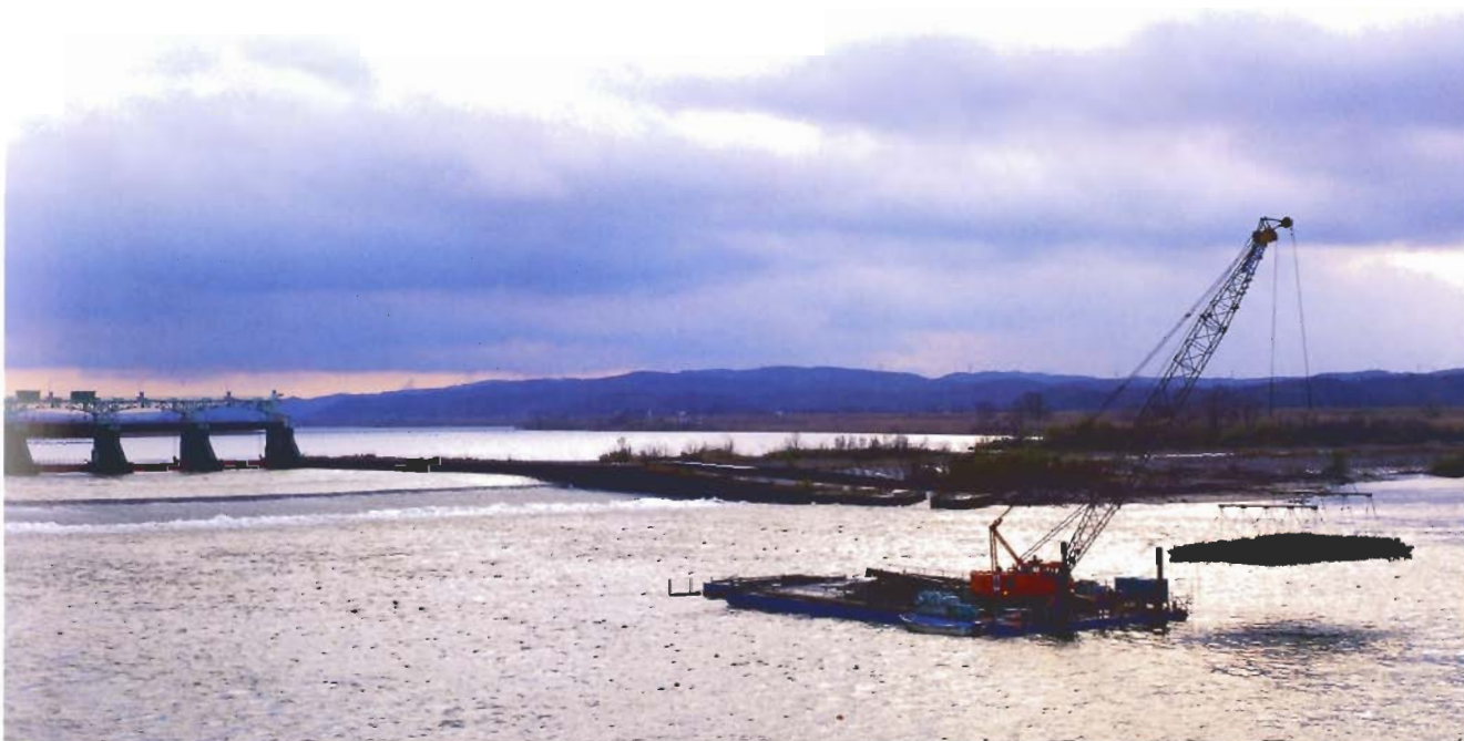
An erosion control mattress made of bundled and latticed branches of various trees, packed with rocks. This traditional construction method was brought to Japan from Holland in the late 19th century. The mattress helps to prevent flooding and provides a tranquil habitat for many water-dwelling plants and animals. (Shinano River, Niigata Prefecture) (Photo: Osamu Nobuhara/FRONT)
