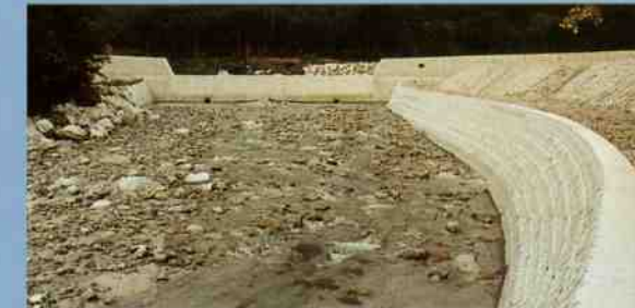
尾白川第二砂防えん堤 Ojiragawa No.2 Sabo Dam 昭和58年10月完成。高さ7.5m、長さ133.0mの重力式コンクリートえん堤。 It was completed in Oct., 1983. It is a gravity type concrete sabo dam with 7.5 m of the sabo dam height and 133.0 m in length.
