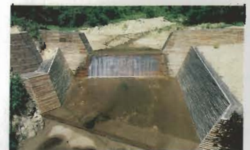
Nirenoki-sawa ground sill work No. 1 has a wooden surface to ensure harmony with the surrounding landscape.
